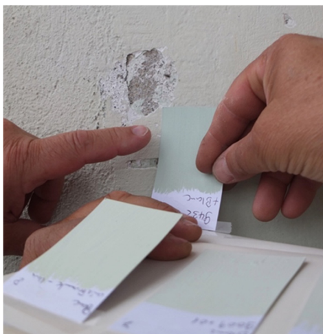
Fig. 5 Stratigraphic survey and essay of painting for the façade of the Petite Villa, 2012 © FLC.
