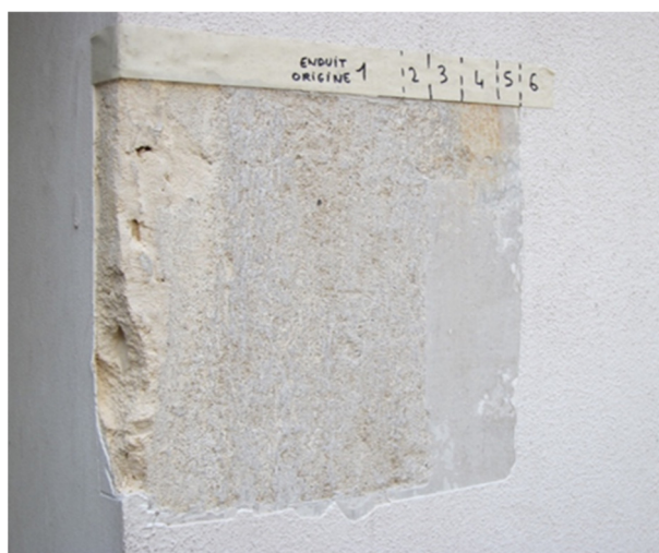
Fig. 4 Stratigraphic survey on the facade of the Maison La Roche: in layer 1 the original plaster (Cimentaline).
